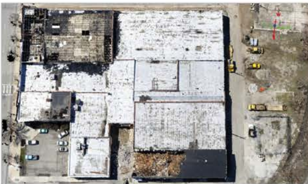
Woolpert uses UAS data to monitor construction as well as demolition. Above is a point cloud showing how demolition is progressing at a jobsite. Courtesy of Woolpert
