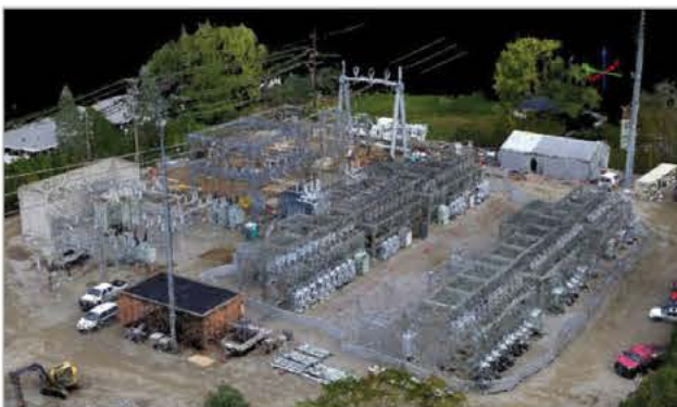
Woolpert used an unmanned aircraft system (UAS) to collect this colorized point cloud of a utility substation. Woolpert has used UAS in more than 100 projects since 2014 to collect data, monitor construction, verify safety issues, explore remote and tight locations and support airport asset management programs. Courtesy of Woolpert
