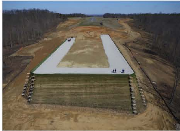
UAS data is being used to monitor the progress of construction on a runway extension, allowing stakeholders from different locations to watch as the project advances. Courtesy of Woolpert
