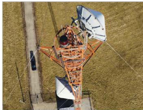
Woolpert uses high-resolution imagery to inspect infrastructure of all sorts, such as this communications tower. Courtesy of Woolpert
