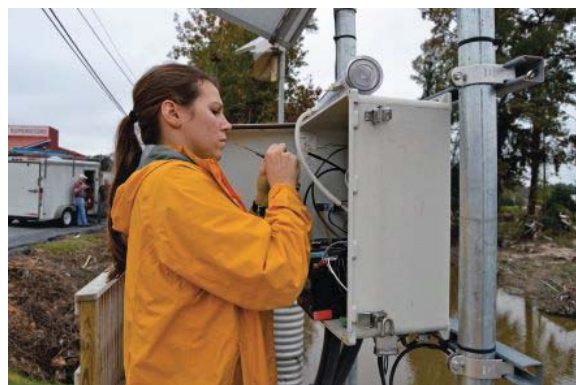
An engineer reconnects a new sensor to the data logger. Each monitoring location contains a Campbell Scientific data logger, a power source, and cellular telemetry, which allows the city to view the data on a website.
