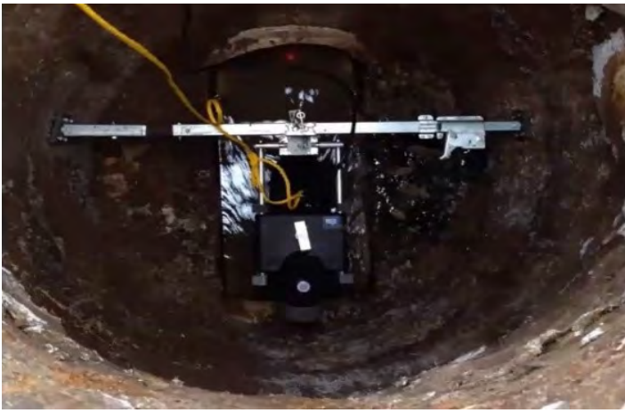
Figure 8: Flow meter installed in a manhole
